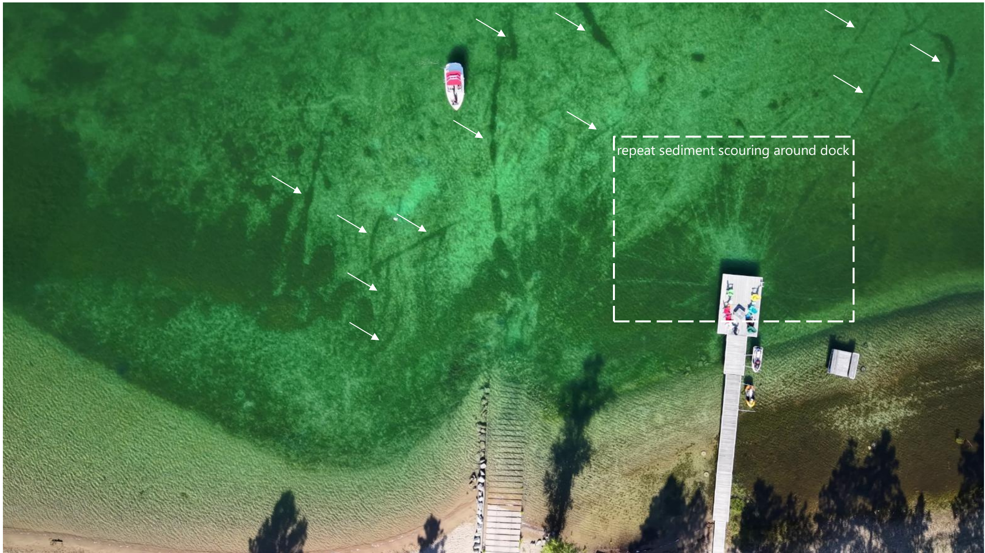
Figure 13: Sediment scouring at Wasa Lake Provincial Park's boat launch, 2025 Note: Arrows and boxes indicate some scours/trenches
